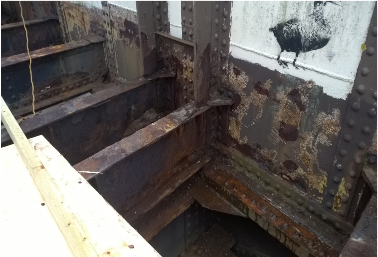
Condition of the main two cross beam at central support pivot area – now replaced
