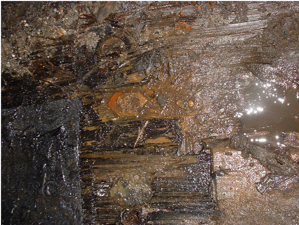
Deteriorated water sodden condition of Timber planking in and around the kentledge end of bridge
