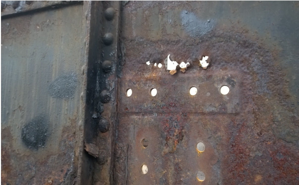
Typical example of loss of main beam web section of main girders
