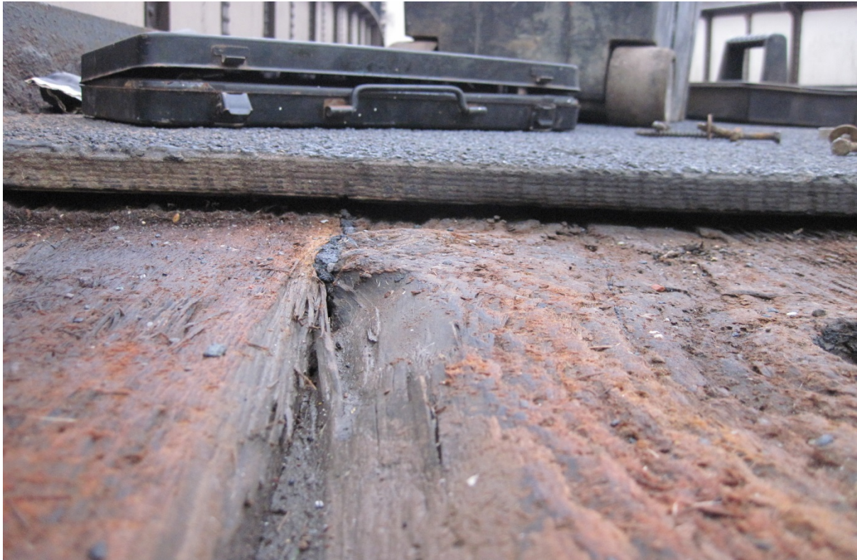
Typical example of decayed timber planking underneath the road surfacing boards
