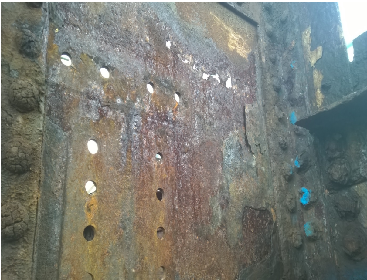
Further example of lost of web section to main girder beams
