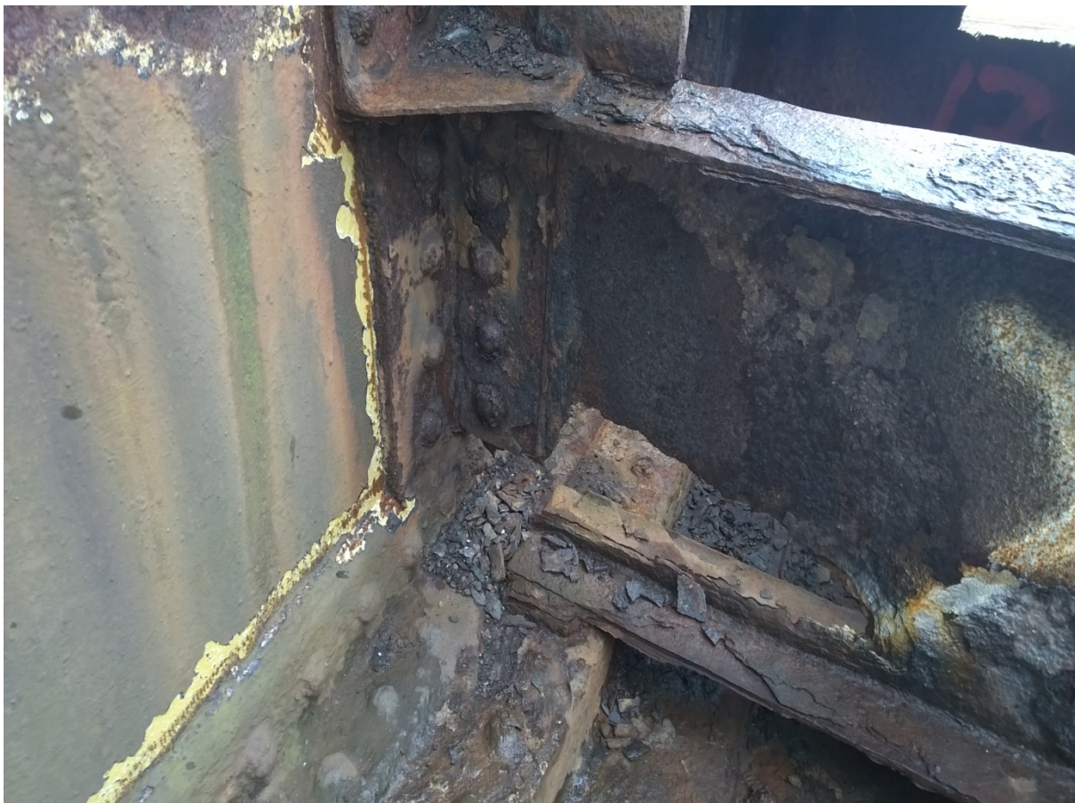
Typical Condition of total cored through cross
