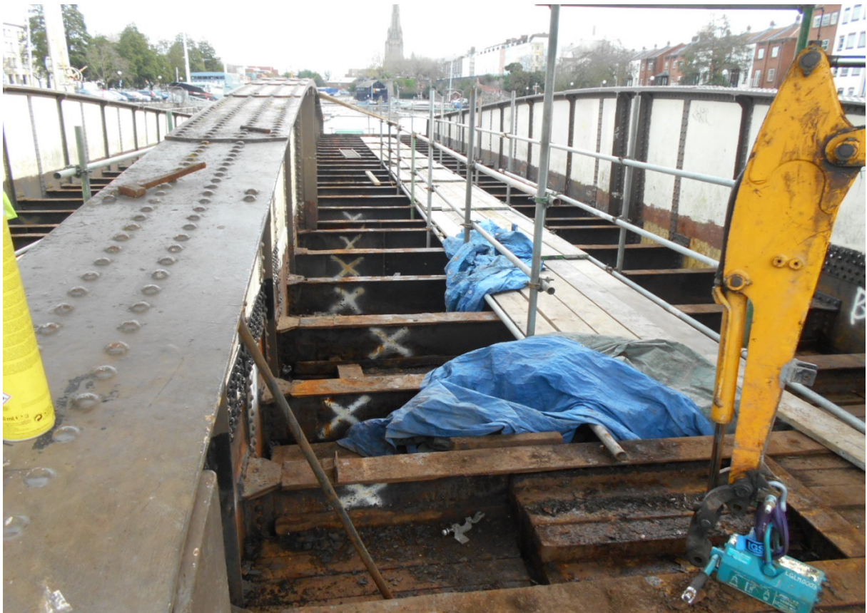
Cross beam (Marked with X) to be removed and replaced with new fabricated bespoke beams
