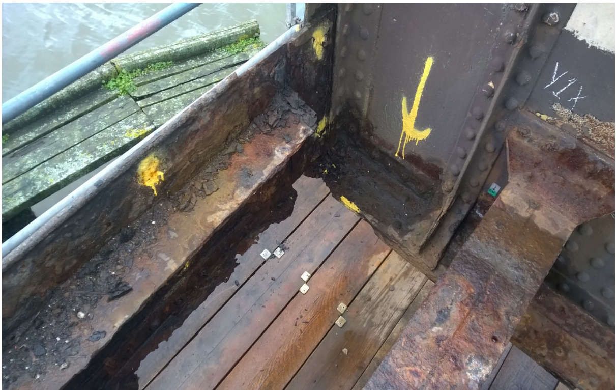
Condition of front curved nose end beam – now replaced
