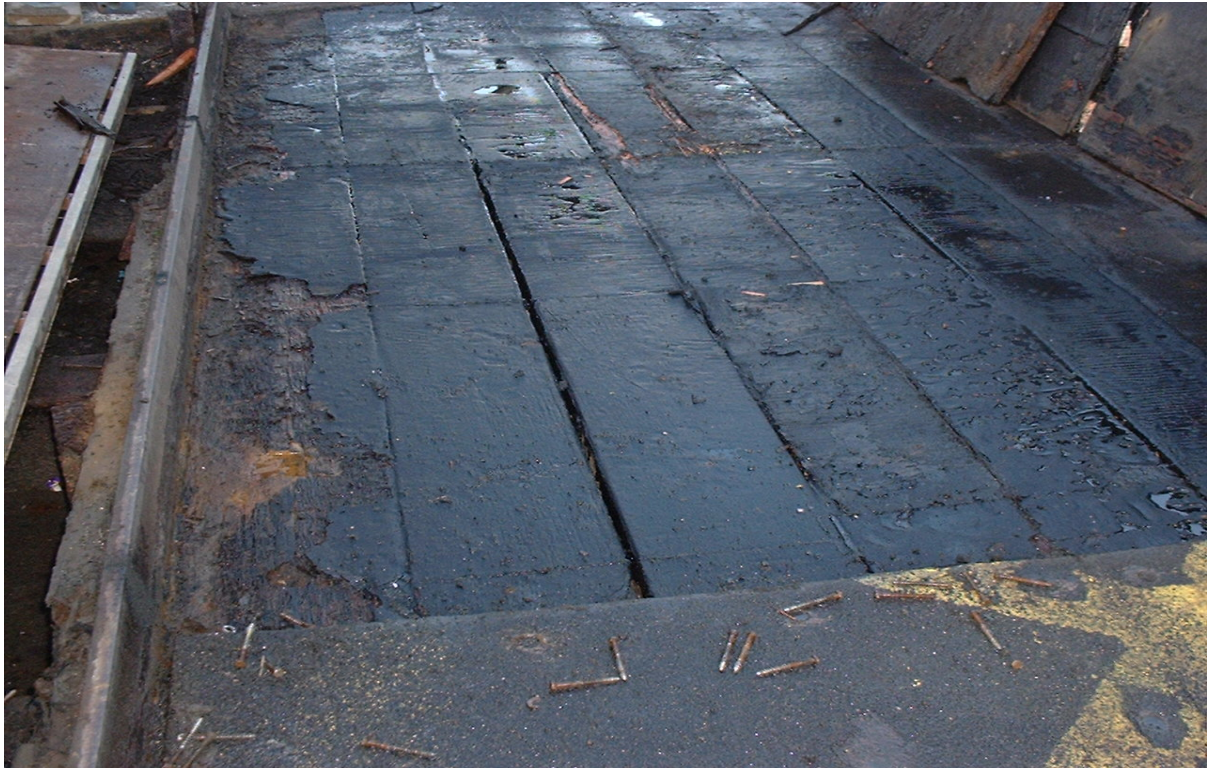
Prince Street Bridge Condition of Timber Plank Decking after removal of surfacing boards
